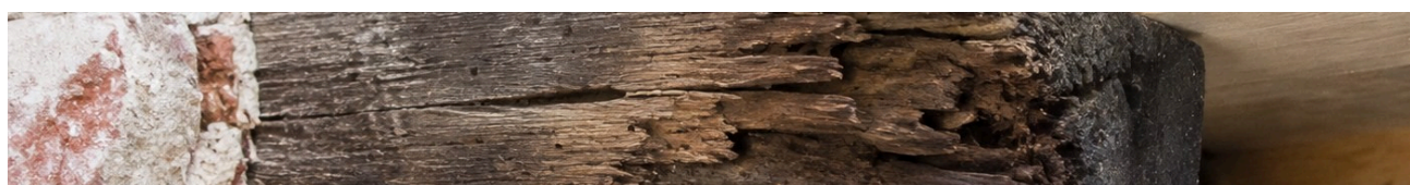
Photograph 9. The same defect further down the curve. By the time it shows internally the structural repair is already necessary.
