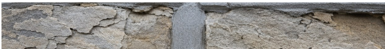
Photograph 1. Cement pointing has not failed. The stone has. The mortar is now harder than the masonry, so movement and salt are relieved through the stone face.
